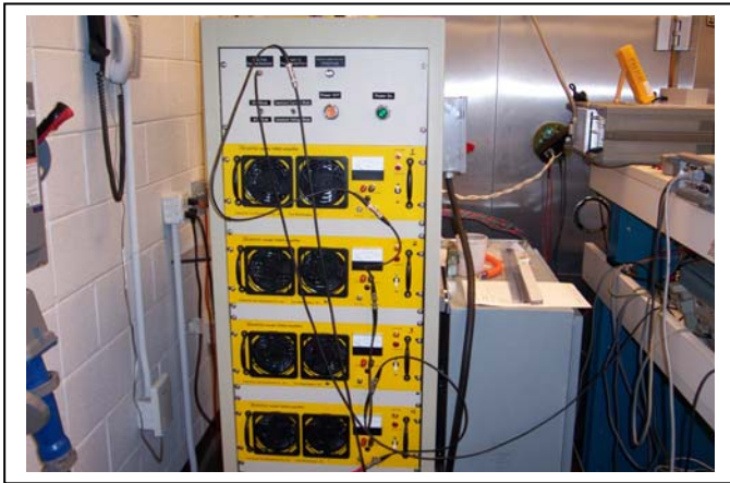
Figure 3. The amplifier stack at ORNL - NTRC
